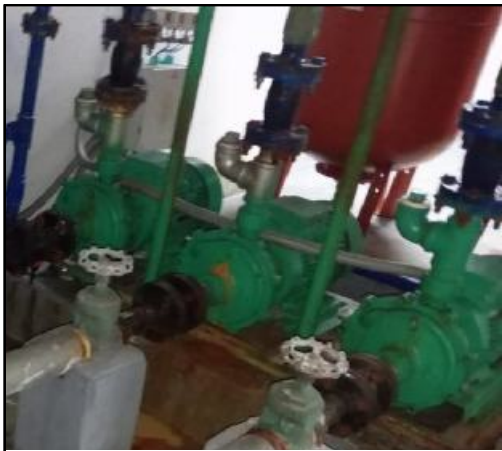
Bombas centrifugas inhabilitada
