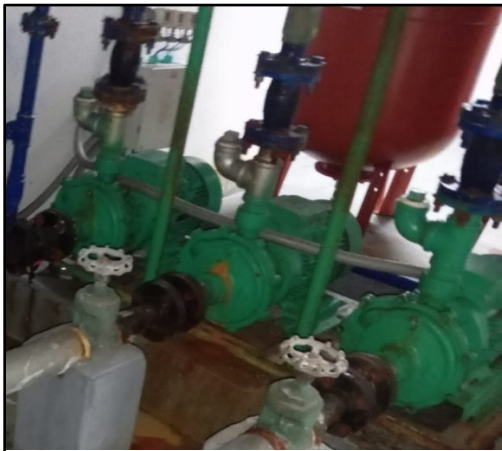
Bombas centrifugas inhabilitada
